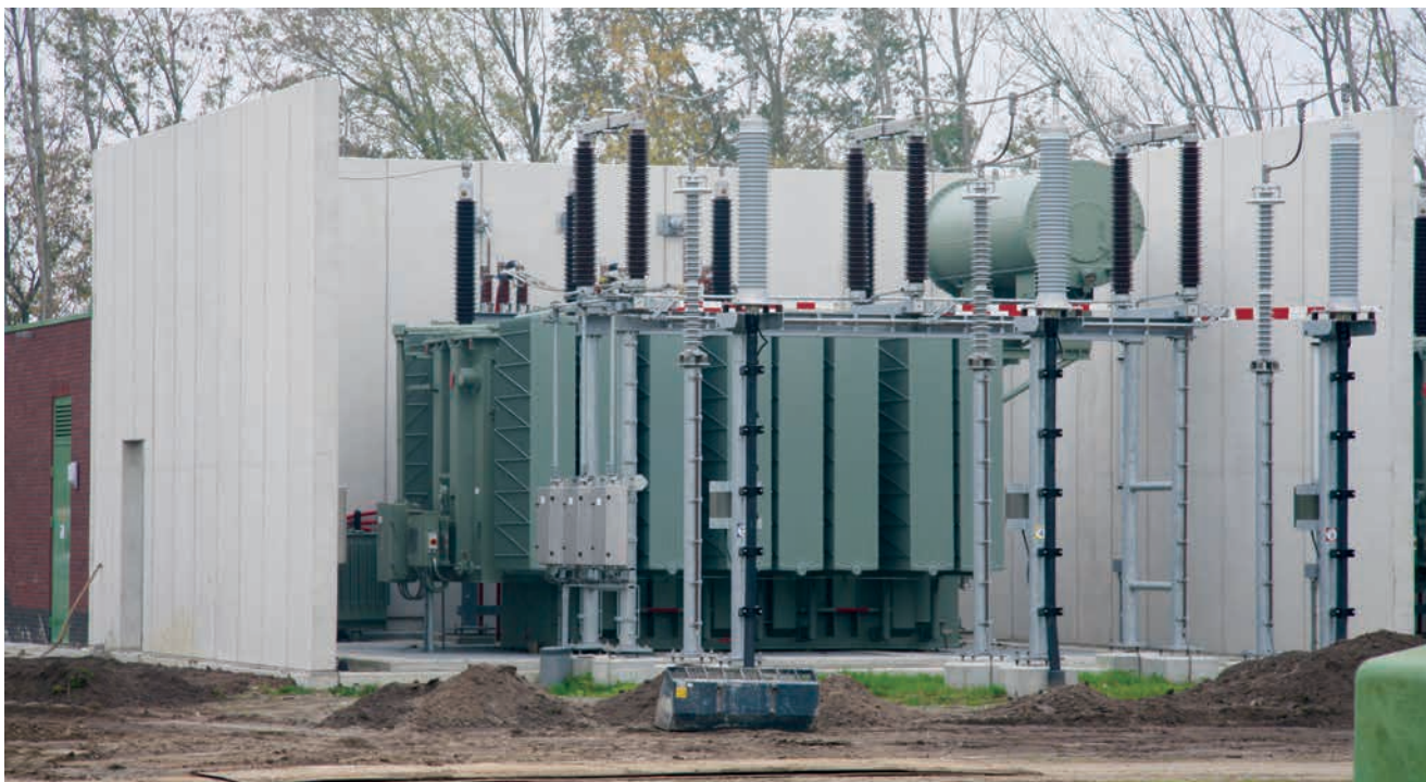
Transformator in U-bak-scherfwand
