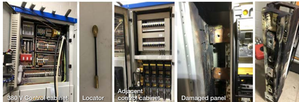
380 V Control cabinet
