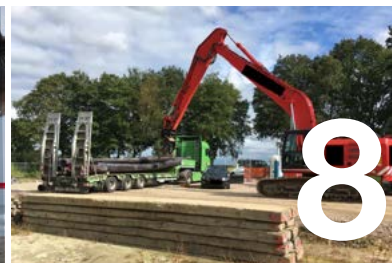
Fatal accident during loading of cable ducts Read more
