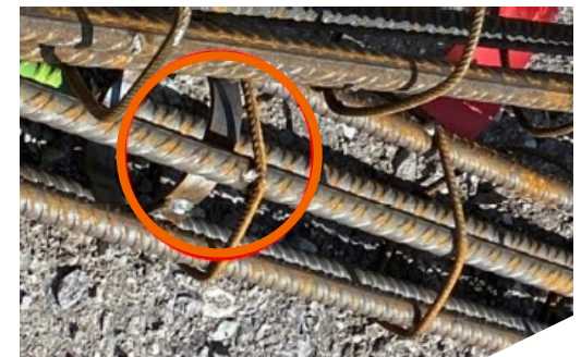
2: Reinforcement cage with torn welded seam at flat bar (attachment point)
