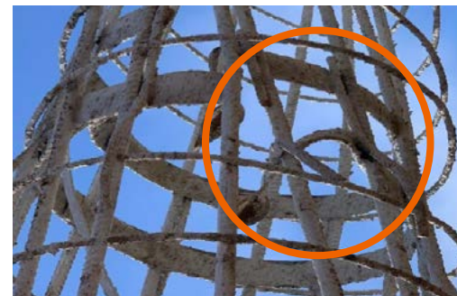
1: Reinforcement cage with cracked flat bar (attachment point)
